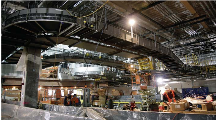
The baggage sortation system at Raleigh-Durham International Airport's Terminal 2. An in-line baggage screening system allows the airport to integrate Explosive Detection System machines, normally seen in airport terminal lobbies, with an airport's behind-the-scenes baggage handling conveyor system. The in-line baggage screening is fully integrated into the airport's baggage handling system.
